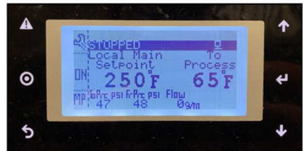
Advanced PLC Controller
